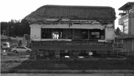
Fig.16: Field Trip on March 14, a damaged heritage building in Kesennuma city (Photo by Randolph Langenbach)
